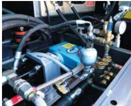
Water high pressure system
