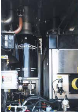
UL listed boiler
